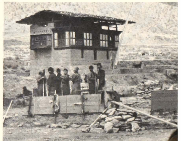
5. Shops under construction, farmhouse behind. The earth wall is being rammed by women.
